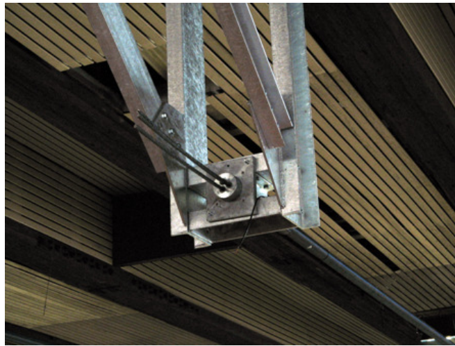
Fig. 12 Anchorage of the Cable Tie Rod to the Steel Brackets
