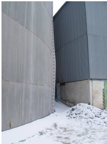
Fig. 6 Local Deformation at the Damaged Location of Silo PC2
