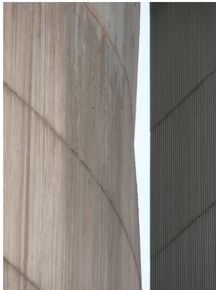
Fig. 5 Local Deformation of Silo PC1 Shell
