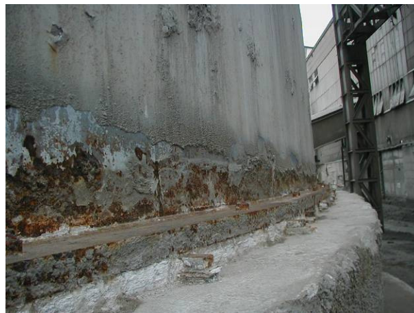
Fig. 4 State of the Shell in Contact with the Base Plate
