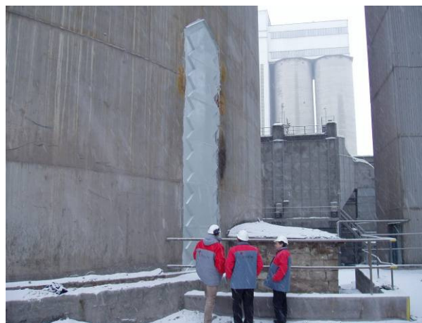
Fig. 3 View of the Finished Repair at the Damaged Location of Clinker Silo PC2
