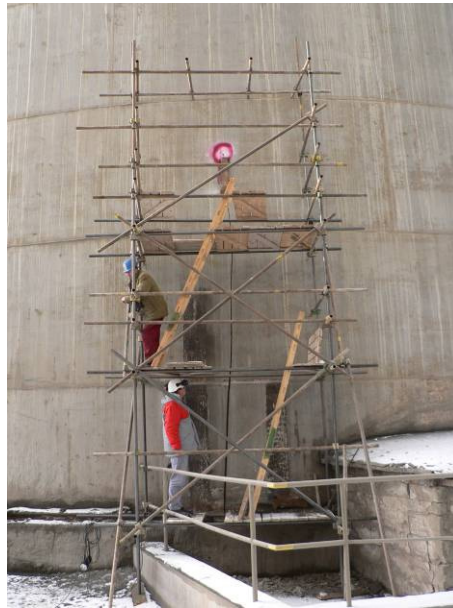
Fig. 2 View of the Crack in Silo PC2 (November 2005)
